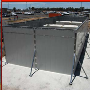
(Mining camp power station enclosure)
