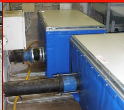
(Acoustic covers on pumps)
